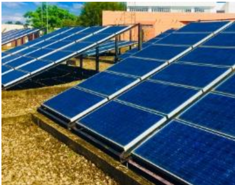
Figura 10: Painéis SX 120 U – LABSOLAR/UFJF
