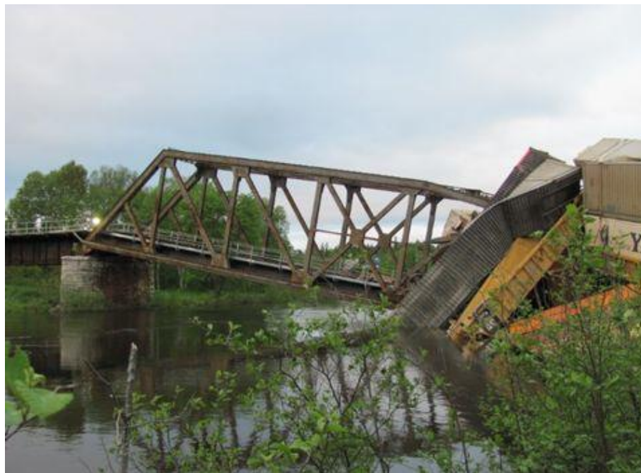
Figure 1 – Collapsed south end of the railway bridge (TSB, 2013).
