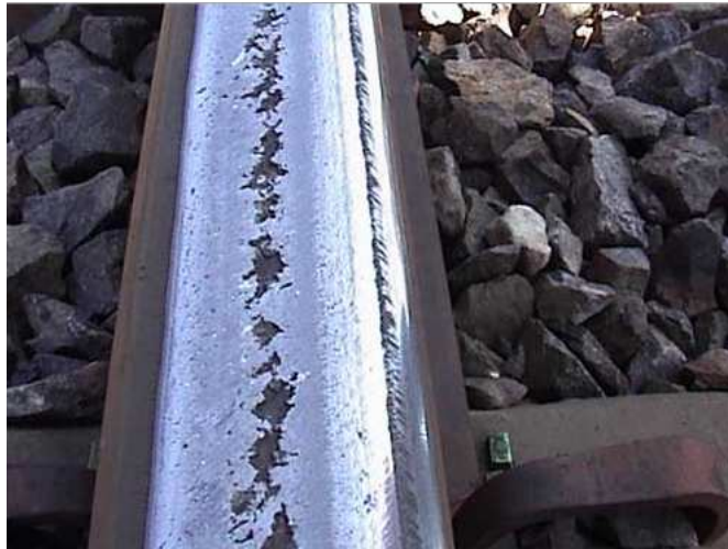
Figure 2: A typical rail head defect.
